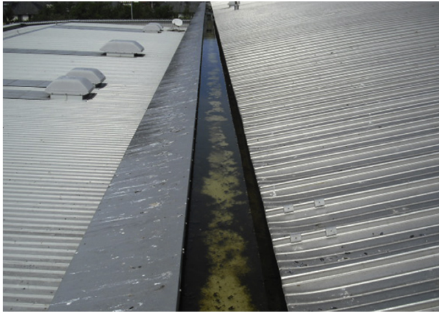
Figure 4.14 Pooling water mixed with bird droppings. Once the roof starts to leak, rain water contaminated with high amounts of pathogens may infiltrate to the inside of the food factory. Courtesy Reactive Group Services.
