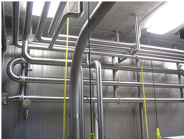
Figure 4.34 Utility piping should be set off the wall for better cleaning. Pipe hanger suspension rods should be smooth and round, and suspended braces should be round tubing sealed at the ends. Cables drop from the ceiling, hence reducing the risk of contamination. Courtesy of CSI Central States Industrial, www.csidesigns.com (Moerman, 2011c).
