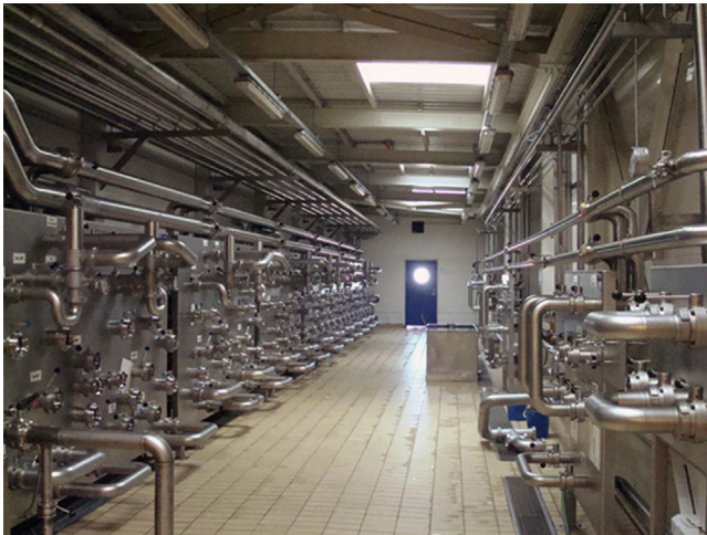
Figure 4.22 Some of the operative work is relocated from the dry zone H preparation/decontamination areas to the zone H transfer station room where wet cleaning is applied. Courtesy of FRİĞO MEKANİK & PANEL SİSTEM A.Ş.
