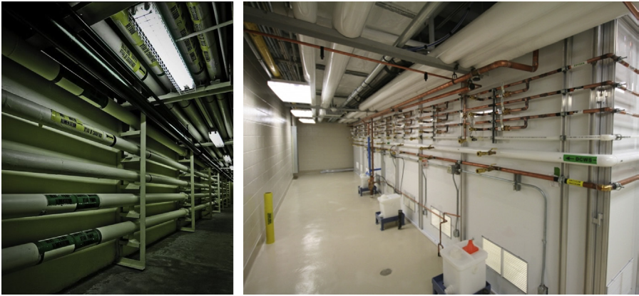
Figure 4.51 Utility piping placed in a technical corridor.
