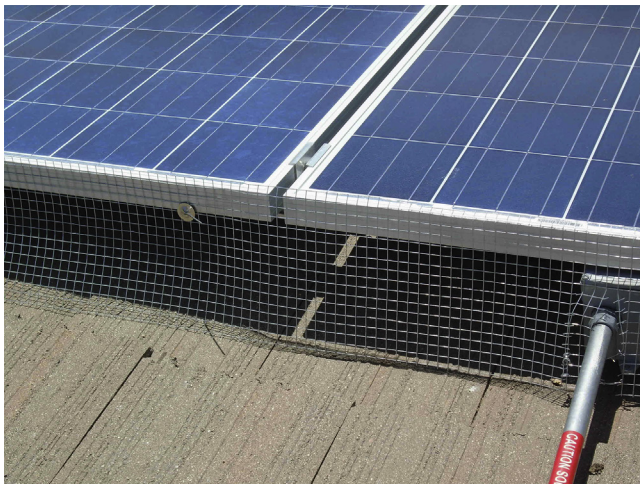
Figure 4.16 Wire mesh systems can keep all birds from getting under solar arrays. Courtesy Bird B Gone, Inc.
