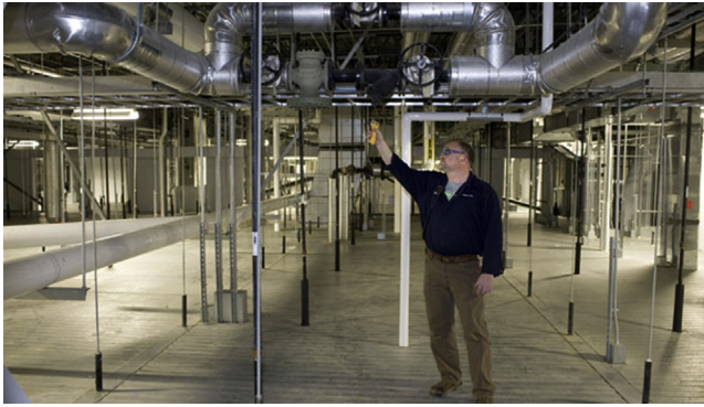
Figure 4.47 The cost of structural steel needed to build a walkable ceiling where personnel can stand erect for easy maintenance discourages some companies from including that feature, but the long-term efficiencies will make it standard within 10 years, at least for pumpable foods. A walkable ceiling has as advantage that maintenance personnel can access the technical area without special gowning.
