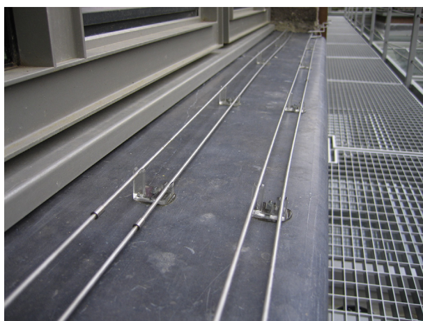
Figure 4.18 Electric bird deterrent system. Courtesy of Kusters Bird Control BVBA.
