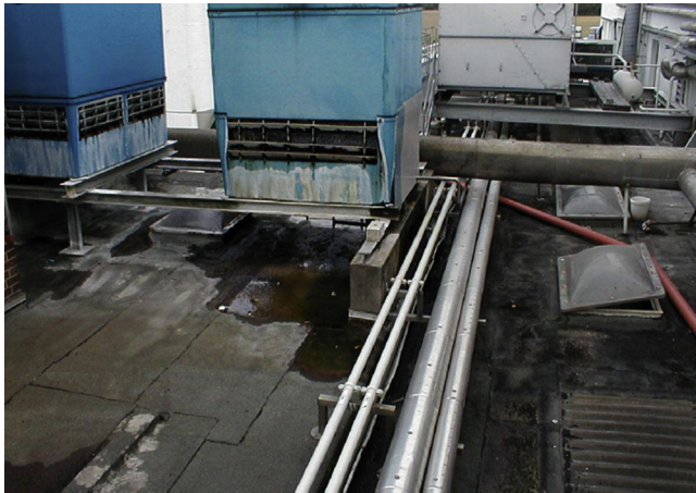
Figure 4.9 Nonweather and water-proof asphalt roof. Liquids may leak to the inside through the many crevices in the asphalt barrier. The roof does not allow adequate drainage and cleaning. Roof openings are unscreened, permitting ingress of rain, debris, and pests. Many horizontal ledges may provide an optimal platform for nesting of birds, and the cluttered installation of utilities makes it easy for rodents to hide (Holah et al., 2014).
