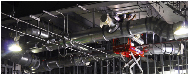
Figure 3.6 Keeping protective caps on open ends of the HVAC ductwork will help prevent dust and dirt generated on the jobsite from accumulation in this ductwork.
