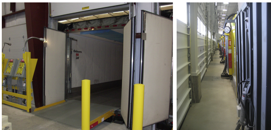
Figure 4.12 Dock doors with leveler plates, which can be raised or lowered to match the height of vehicle loading beds. Factory floor level is a few centimeters above dock floor level. The trailer doors swing open inside the building to control infiltration of bugs as well as the loss of conditioned air.
