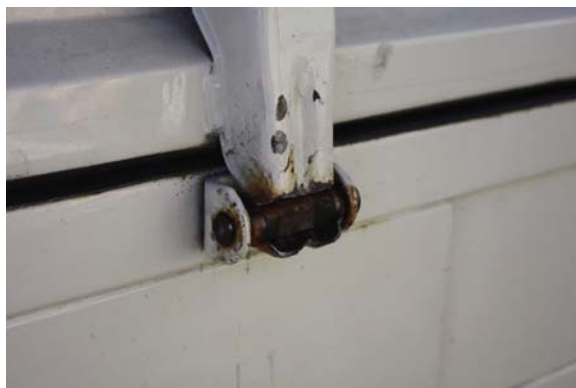
FIGURE 6.12 Paints can crack or peel off.
