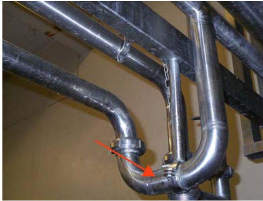
FIGURE 7.28 Nondrainable pipe section. Courtesy of Mondelēz International, © 2016.
