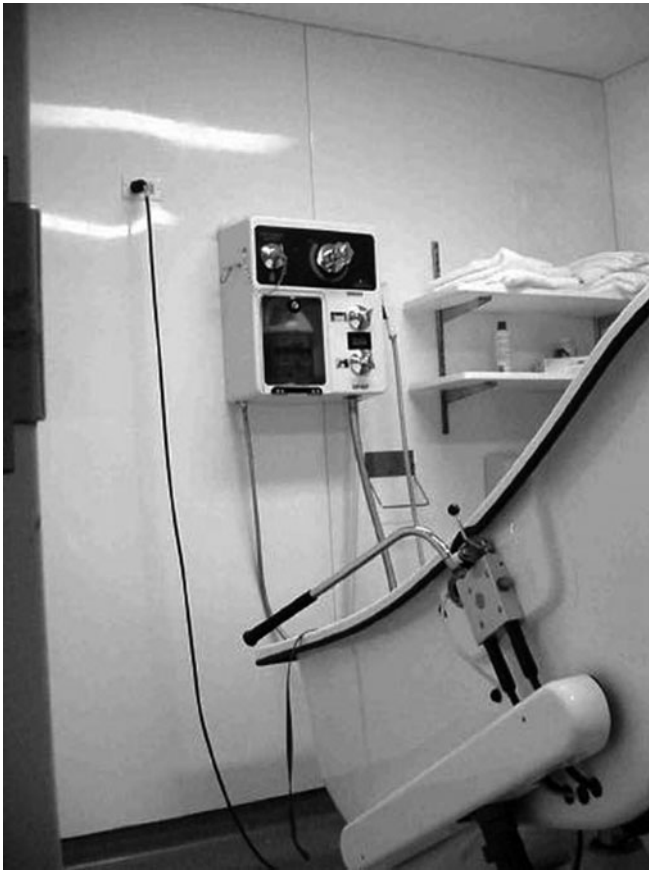
FIGURE 10.2 Undisguised control panel.
